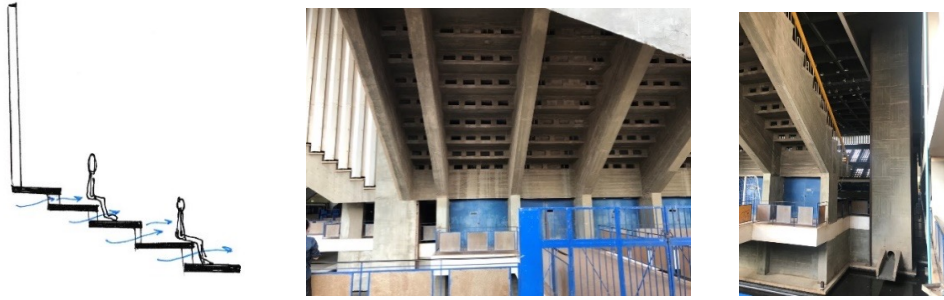
Figure 5 Hole punches underneath of the audience seats provide a soft lighting and ventilation into the indoor arena. Photo by Ty Pisith, March 8, 2018.
